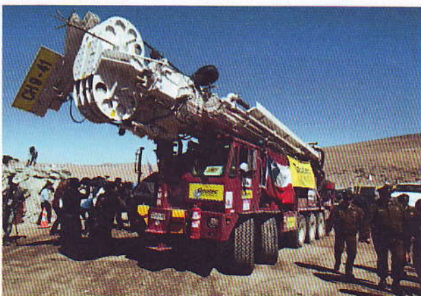
Drill Rig nicknamed "The Miracle" arrives on site in Copiapó, Chile to drill shaft that ultimately rescues the 33 trapped miners.
